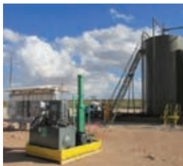
Bottom, left and right: Hydraulic Beam Gas Compressors (HyBGC).
