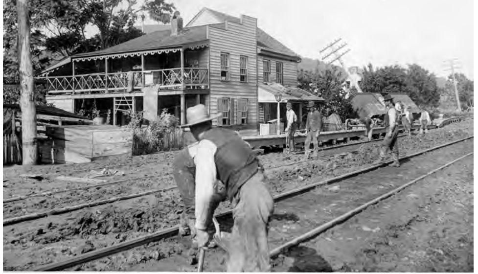
✧ Although it expanded throughout the nineteenth century, the railroad was sometimes impacted by natural disasters. In this image, men clear the railroad tracks in Point of Rocks of debris following a major flood in 1889.
