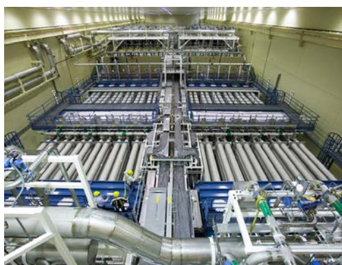
Figure 32.23 National Ignition Facility (CA). This image shows a laser bay where 192 laser beams will focus onto a small D-T target, producing fusion. (credit: Lawrence Livermore National Laboratory, Lawrence Livermore National Security, LLC, and the Department of Energy)
